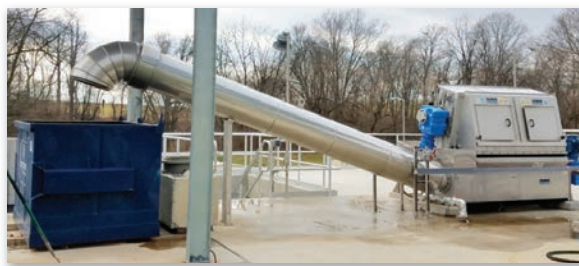
Treatment Plant Bar Screen
