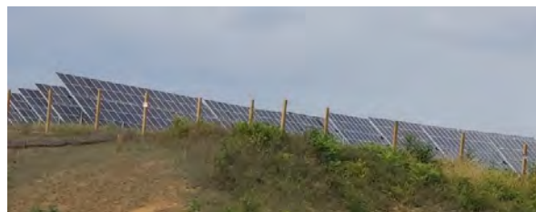
Chambersburg Solar Center – Photovoltaic Panels
