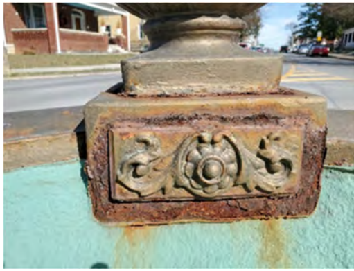
Pre-construction Glen Street Fountain Rust Damage
