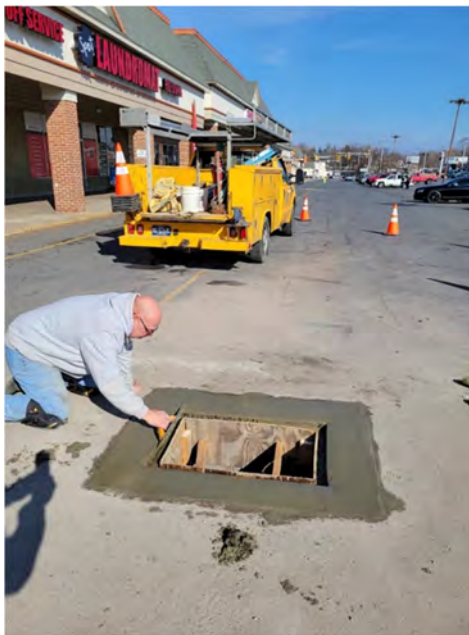
Installing a new storm sewer drain in the Cedar Avenue Right of Way
