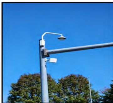
Each traffic signal is equipped with radar detection and a digital 360° camera with a fiber optic uplink to the Borough's traffic management system
