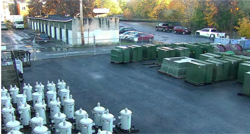
Electric Utility's Transformers and Cable Stored Securely at Warehouse
