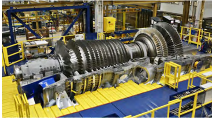
Natural Gas Electric Generation
