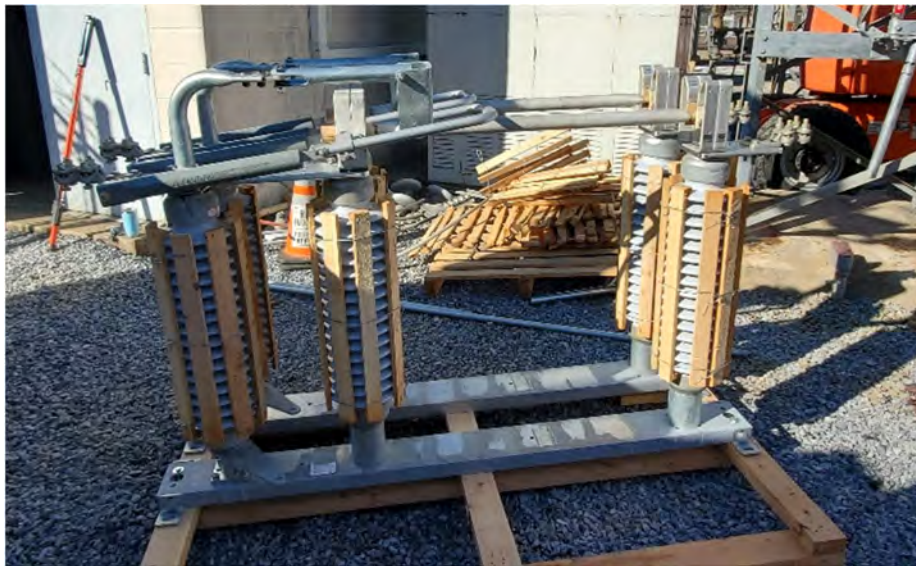
Substation Hardware, Transmission & Distribution, Relay & Control Reconfigurations and Upgrades
