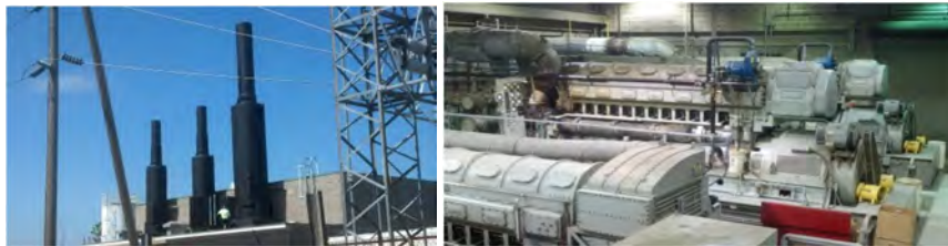
Falling Spring Generation Station - Unit #7 (1999) in Foreground, #6 (1968), and #5 (1968)
