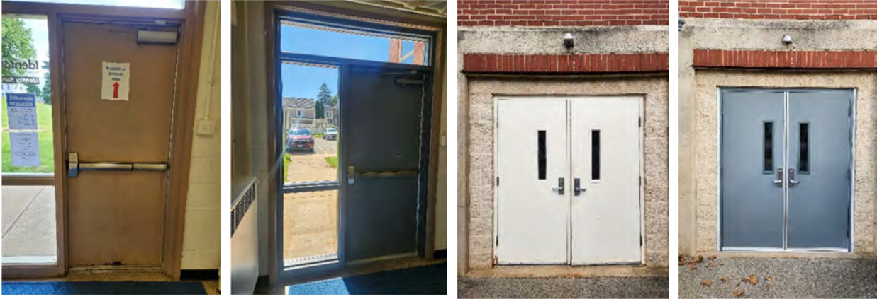
(Before and After) Door Replacement Project at the Rec Center Southwest ADA door; Northwest-most exterior door
