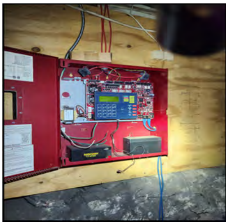
Correcting Basement Fire Violations with the Codes Department
