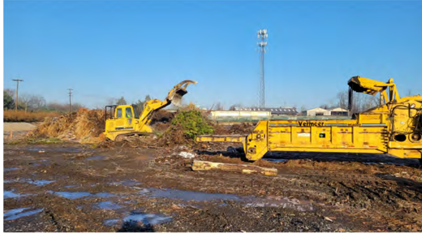
Borough contractor: H & H General Excavating d/b/a Country Boy Mulch & Soil Products
