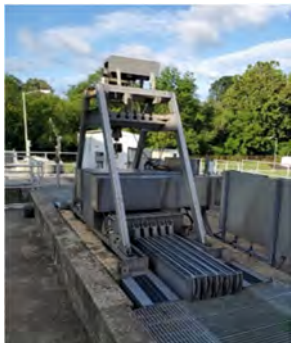
Aging Equipment – UV Disinfection
