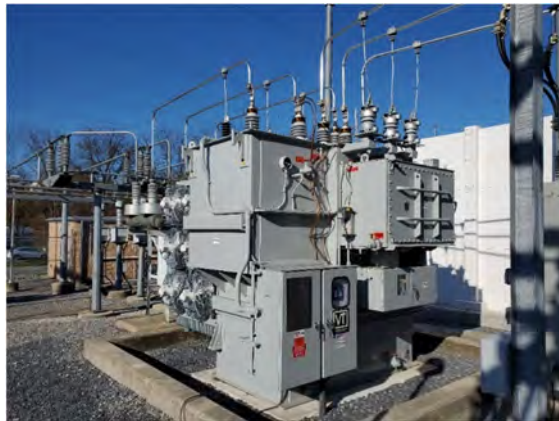
Upgraded Commerce Street Substation Transformers
