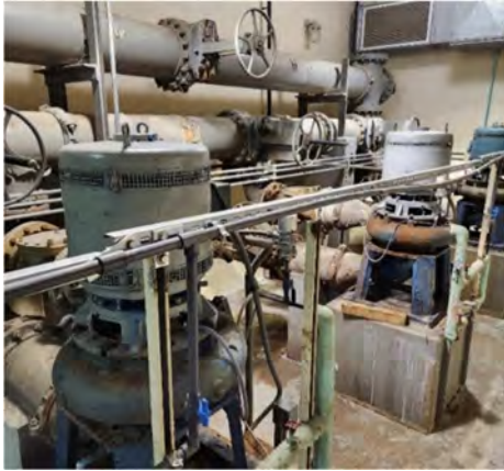
Aging Equipment – Old Headworks
