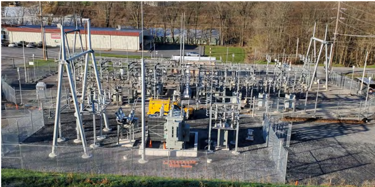
Chambersburg Community Solar Interconnection Substation
