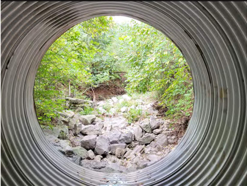
Outfall Pipe To Conococheague Creek
