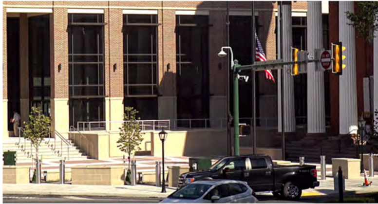
The IT staff is involved with the installation and interconnection of traffic signal and camera to the Borough-wide fiber optic network as depicted in this image of Courthouse Plaza.
