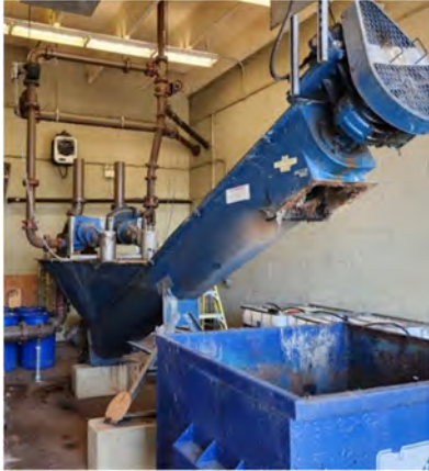
Aging Equipment – Grit Removal
